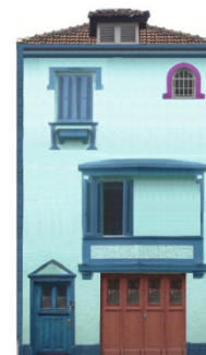
Figure 3: Building 1: historic building with disorder
