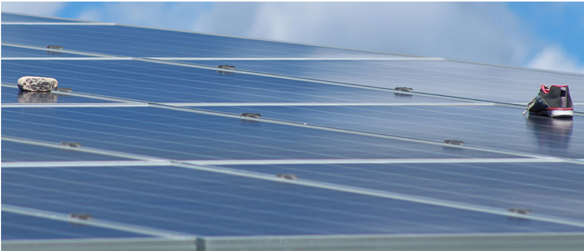
Figure 7. Objects thrown onto solar PV canopy structure in an elementary schoolyard
