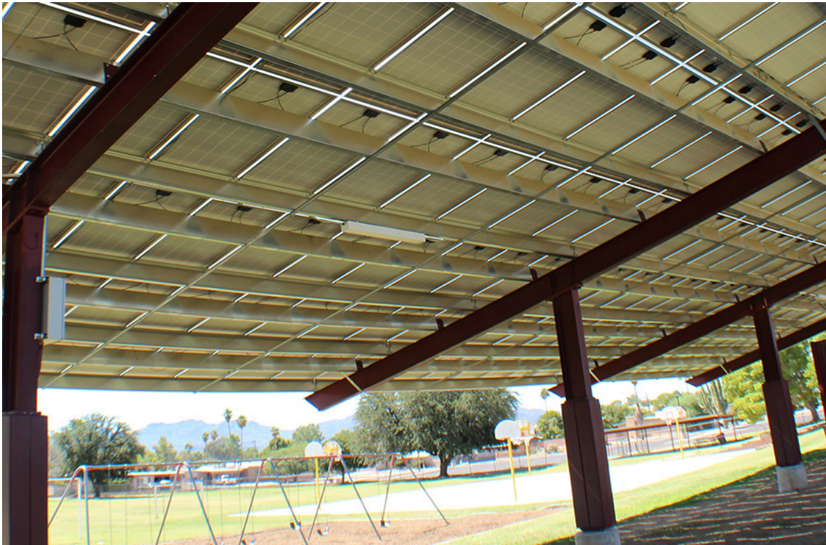
Figure 5. Solar array spanning a public elementary schoolyard
