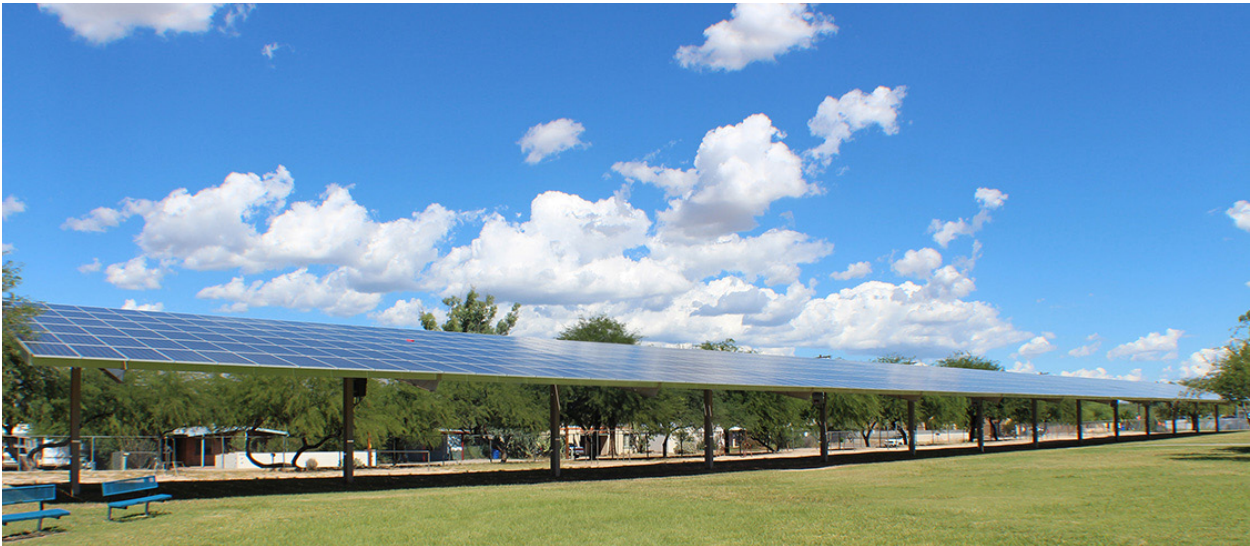
Figure 6. Solar PV array that stretches the length of a schoolyard
